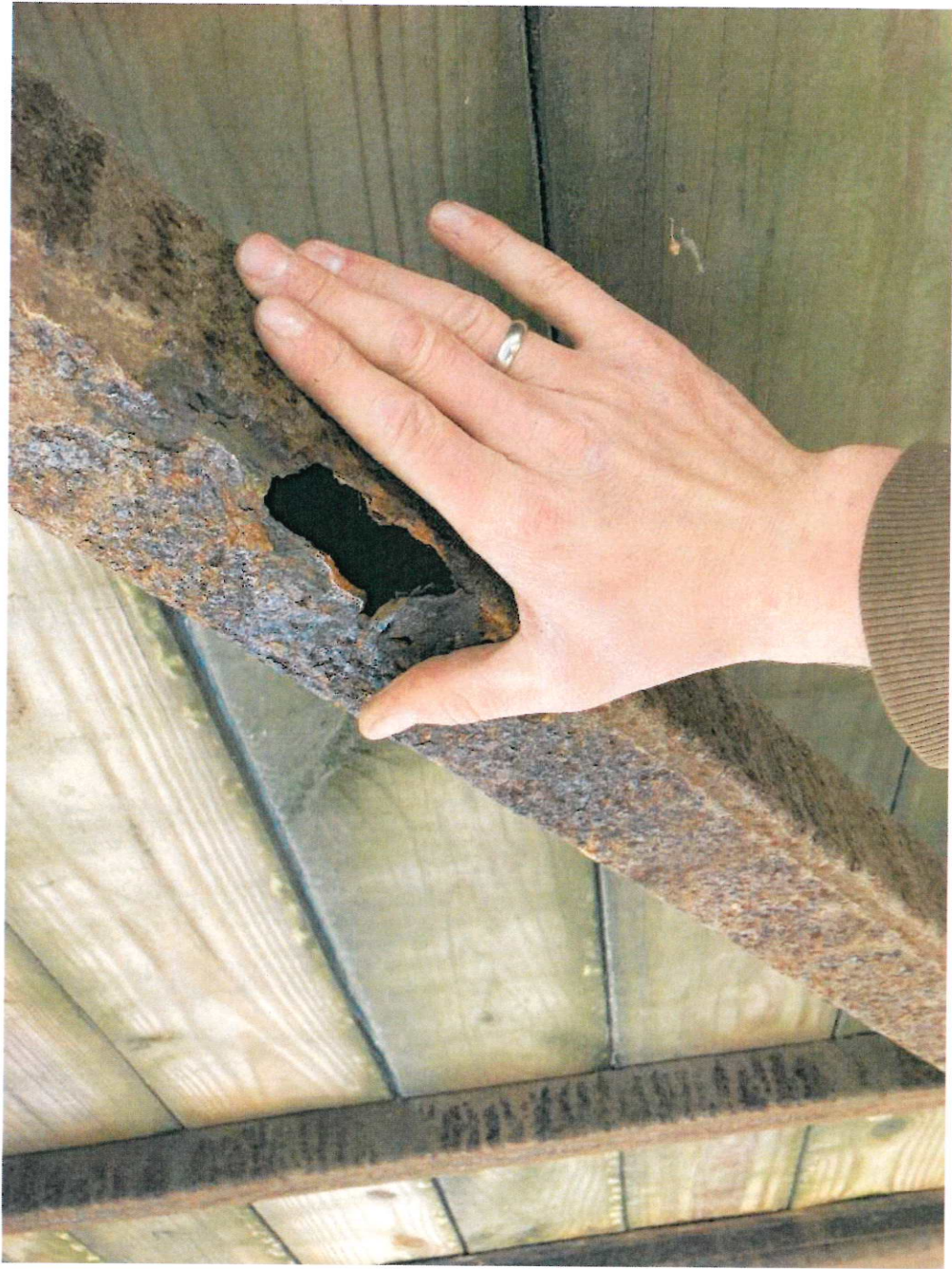
Rec Path Bridge Scoping – Visible Deterioration
