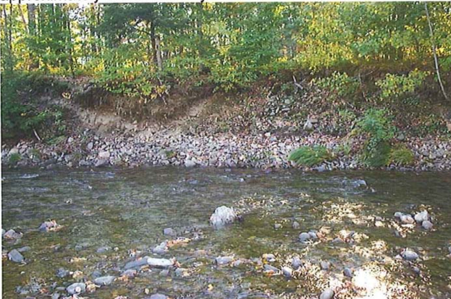
Figure 14. Erosion on Reach 4
