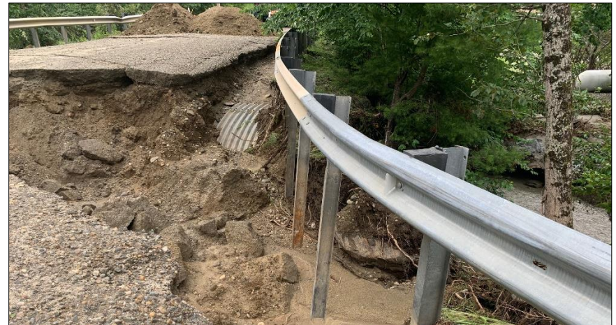
Road erosion impacts from recent flooding event. Photo credit: Town of Stowe
