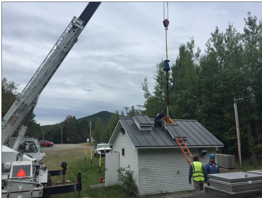
Municipal water pump station. Photo credit: Town of Stowe
